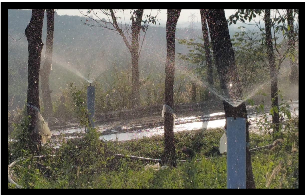
Sprinklers Installed in the project area
