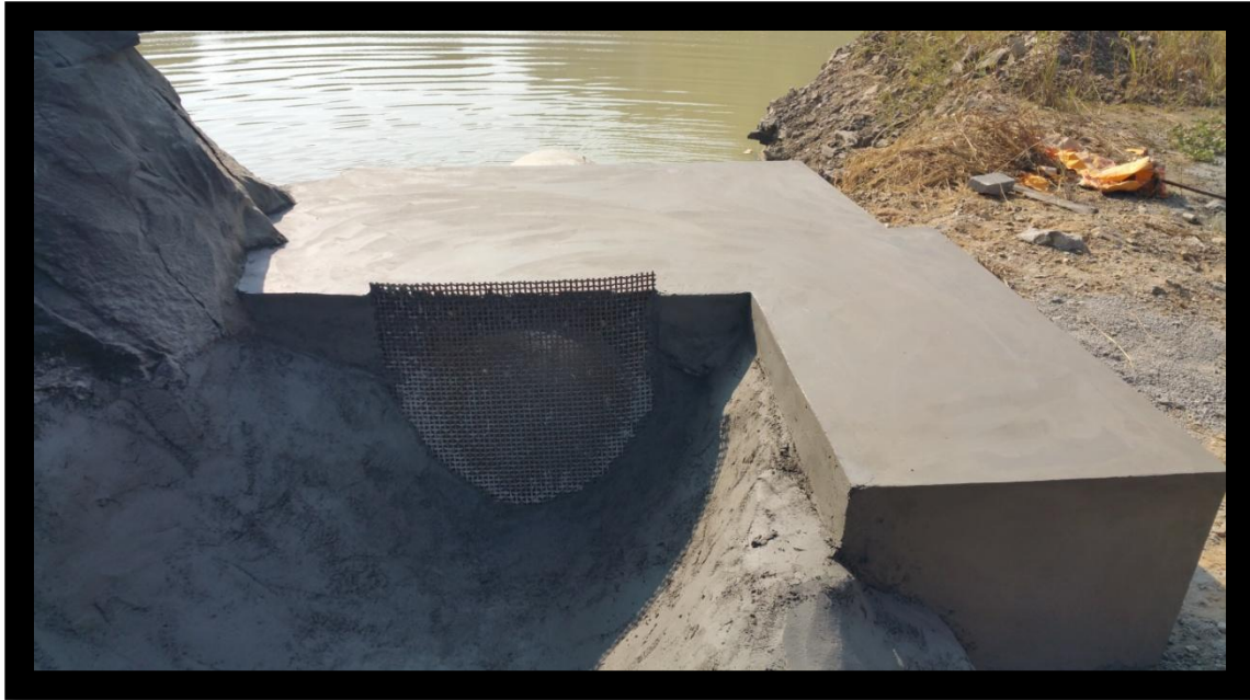
Slit trap to prevent quarry wastes entering in to the main stream
