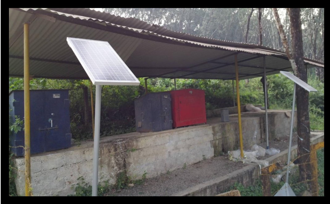
Solar street lights installed near to the magazine
