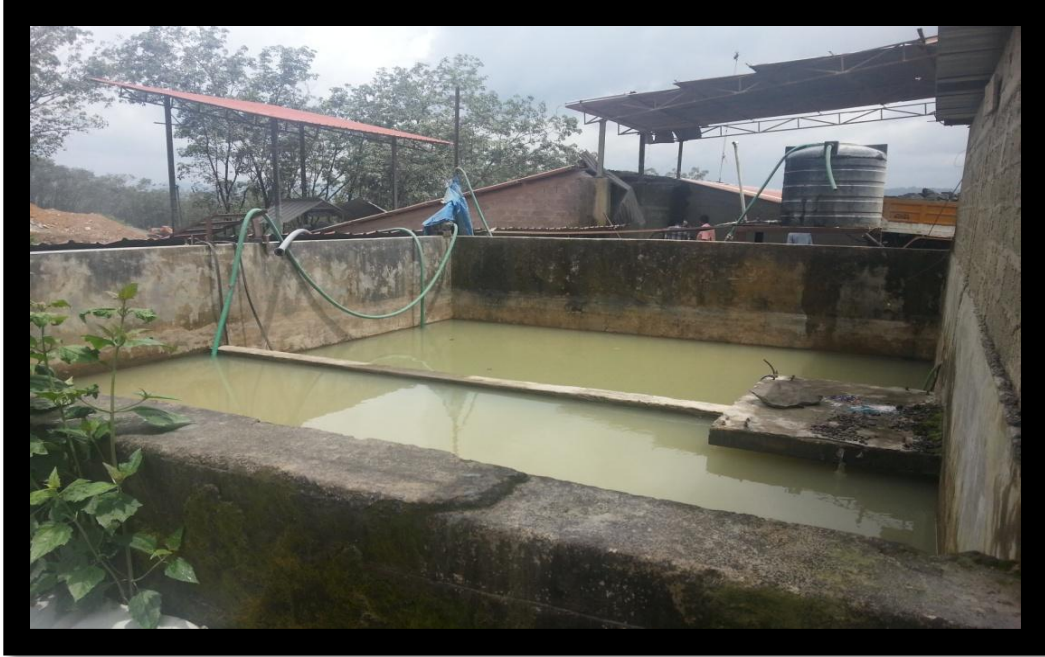
Rain water collection tank
