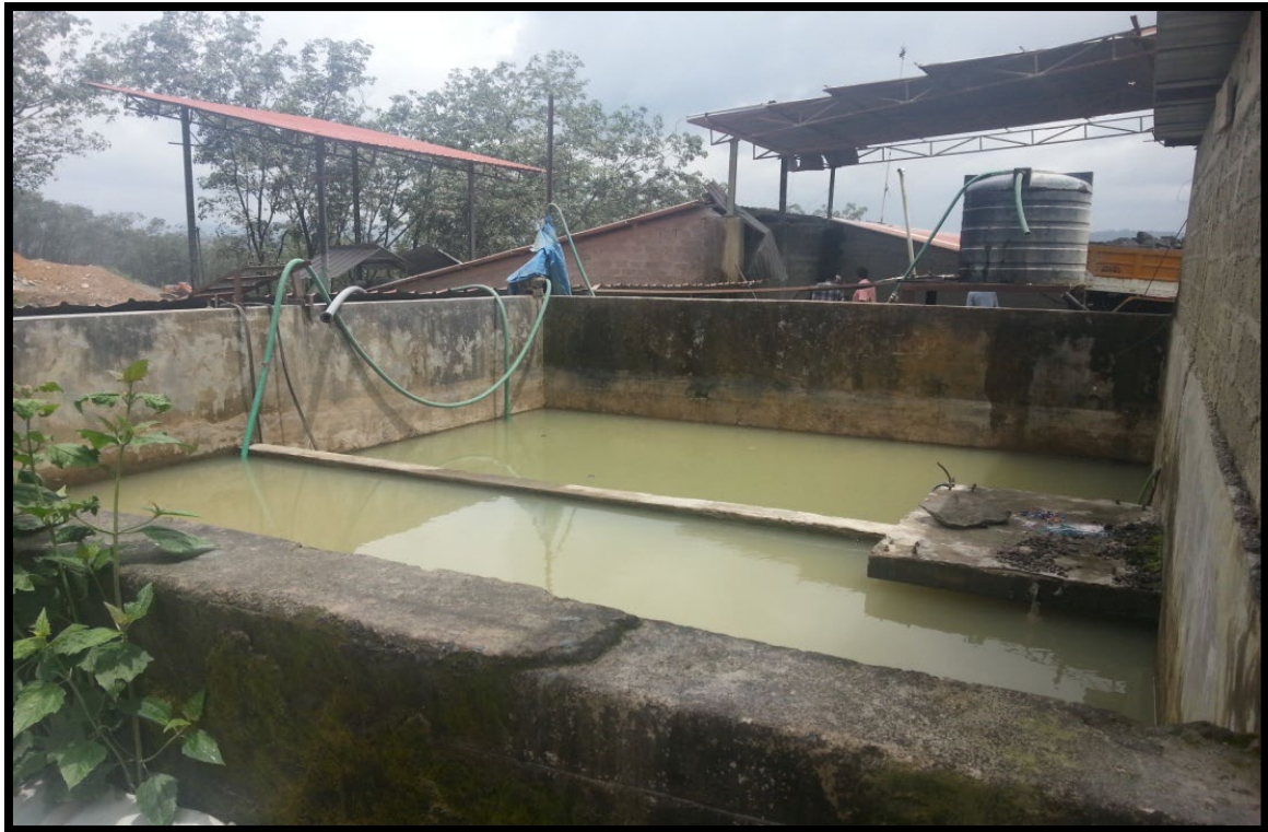
Rain water collection tank
