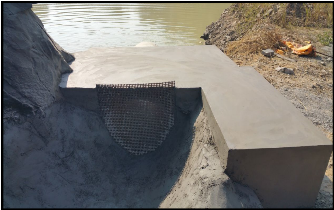
Slit trap to prevent quarry wastes entering in to the main stream
