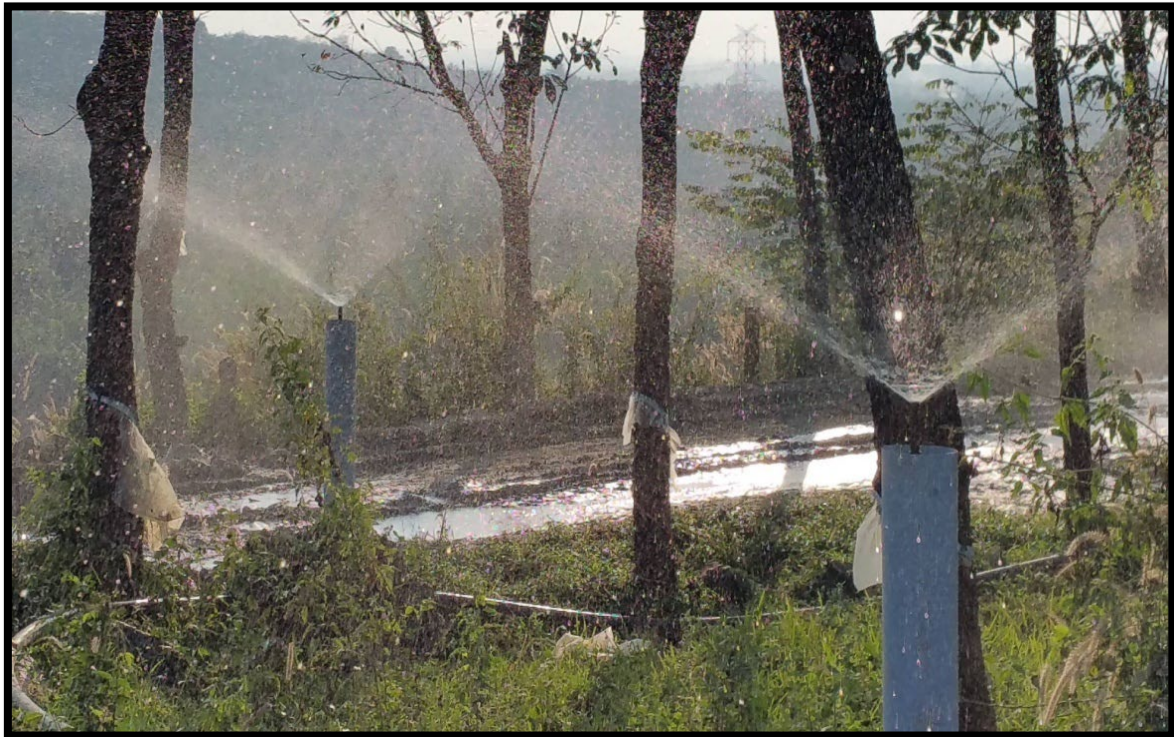
Sprinklers Installed in the project area
